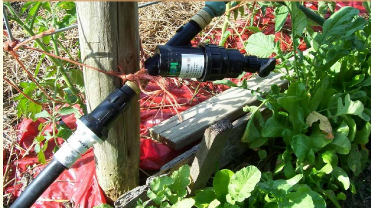
Supply, pressure regulator & filter
