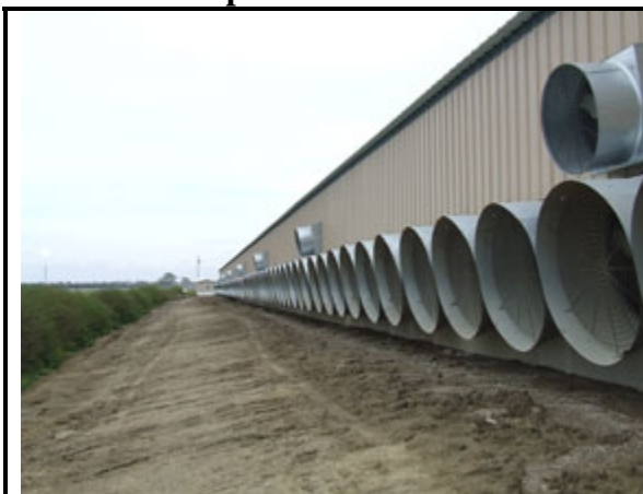
Mechanical Ventilation Freestall Barn
