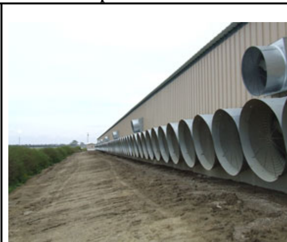
Mechanical Ventilation Freestall Barn
