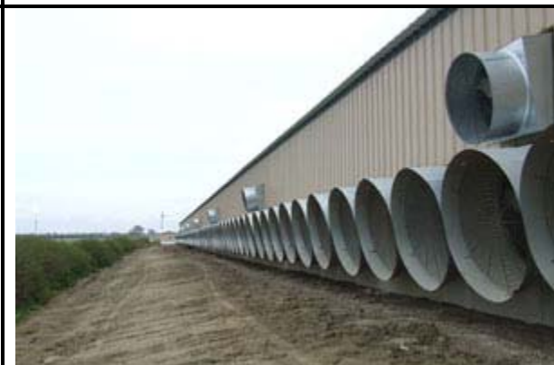
Mechanical Ventilation Freestall Barn
