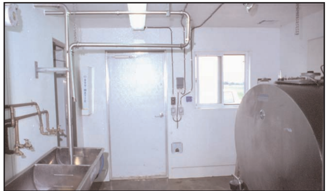
Figure 11.2. Interior of the tank room of a swingline parlor.
