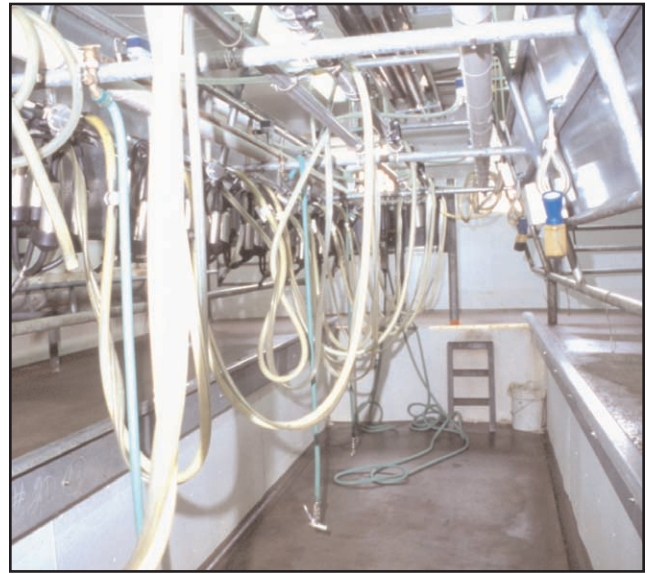
Figure 11.3. View of the operator pit in a swingline parlor.
