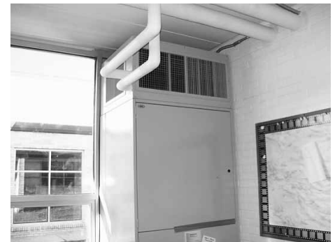
Heat exchangers like this one at Gainesville help to distribute heat evenly throughout the school.
