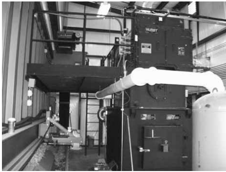
Wood chips are augured from a storage bin onto a conveyor (lower left) to the combustor which sits beneath the boiler (right).
