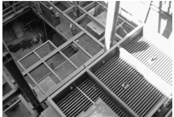
The economizer portion of the new biomass boiler (lower right) is nearing completion. Its job is to use recirculate waste heat from the boiler (to be erected in the open space in the top left) and pre-heat incoming water.
