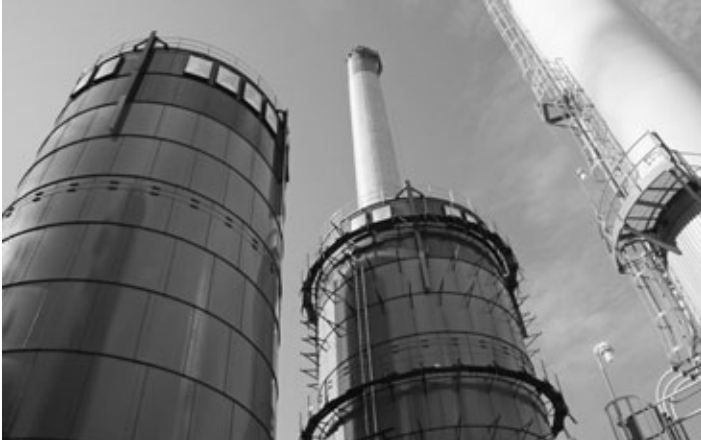
Woody biomass silos are being constructed alongside these newly-built coal storage silos at the MU power plant.
