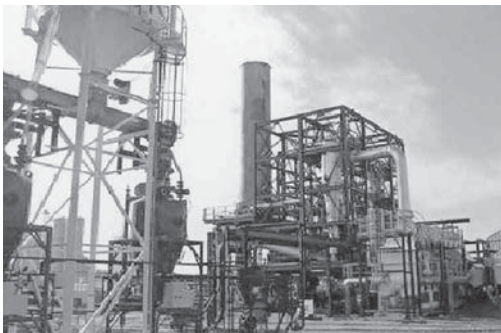
Dynamotive's BioOil plant in Guelph, Ontario
